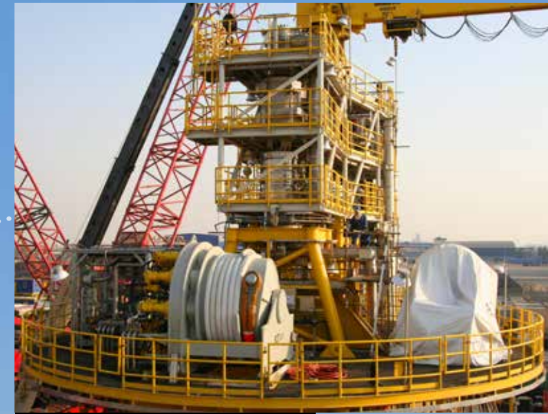
Pull-in / Release Winch in Turret area
